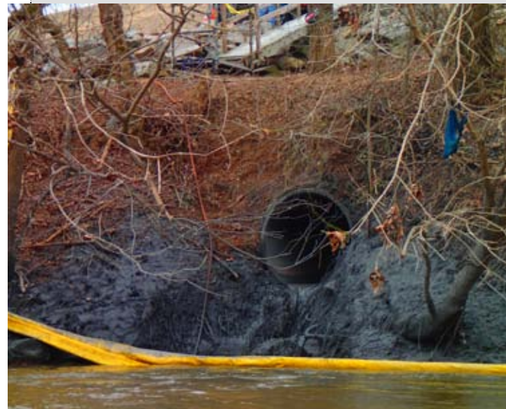
Ash pond outflow pipe. Photo Brian Williams.
