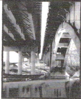
View of construction at Old 87 Bridge south of Eden at 2003 years end.
